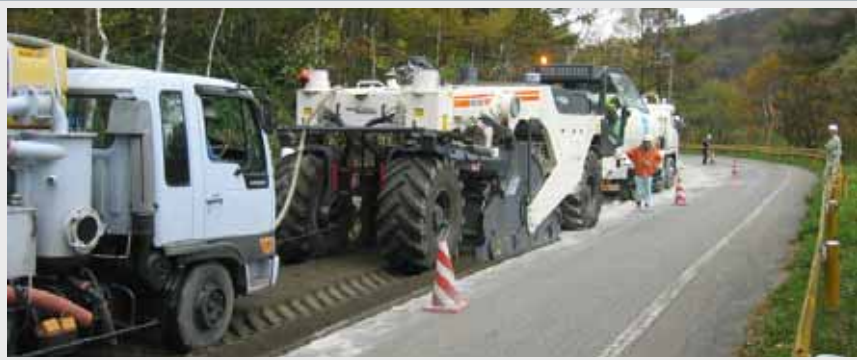
Cold Recycling of the asphalt layer with the Schotterunterbau Working depth 200 mm
