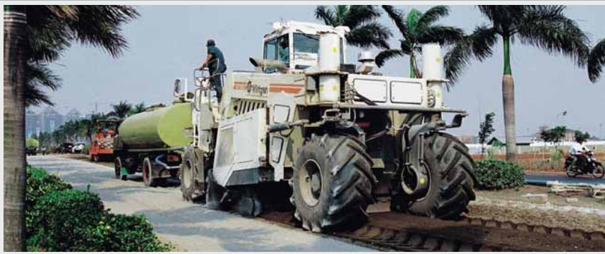
Cold Recycling the asphalt and granular base layers by adding pre-spread cement and bitumen emulsion
