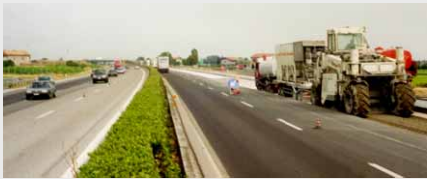
A 14 Milan – Rimini: Rehabilitation of a highway lane - Cold Rrecycling with foamed bitumen and cement slurry -
