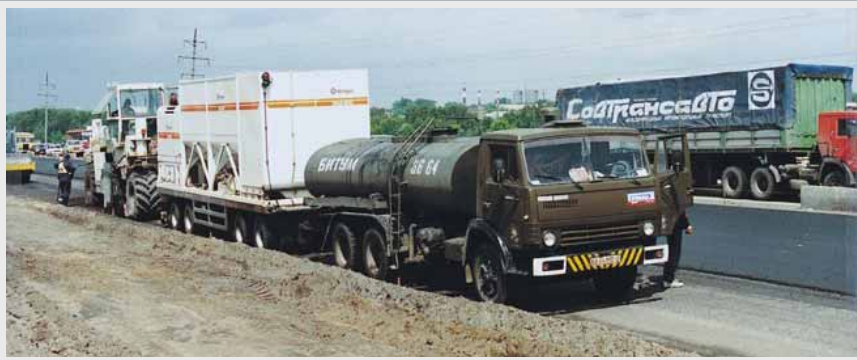
Cold Recycling with bitumen emulsion and cement slurry (WR 2500 + WM 400) Ring Road in Moscow
