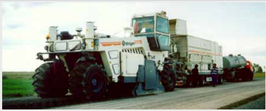
Cold in situ Recycling of a mayor road cement slurry and foamed bitumen: WR 2500 + WM 1000
