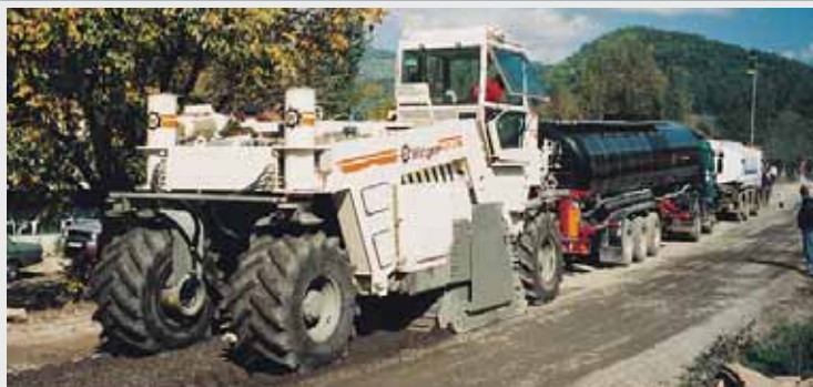
Cold Recycling the asphalt and granular base layers by adding pre-spread cement, water and foamed bitumen
