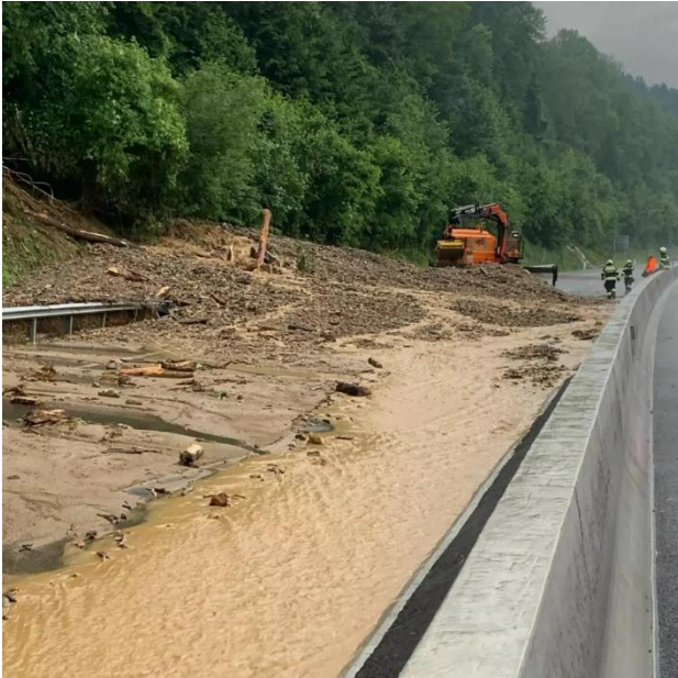
landslide A9, June 2024 (Asfinag)
