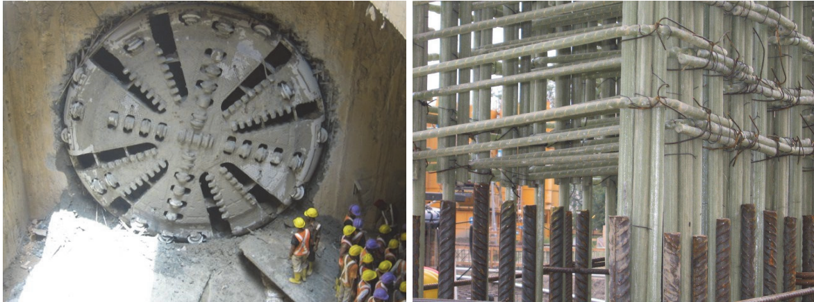
Fig. 8. Soft eye application during the construction of M4 underground line by the Gellért station (Photo: courtesy of Lajos Bán)
