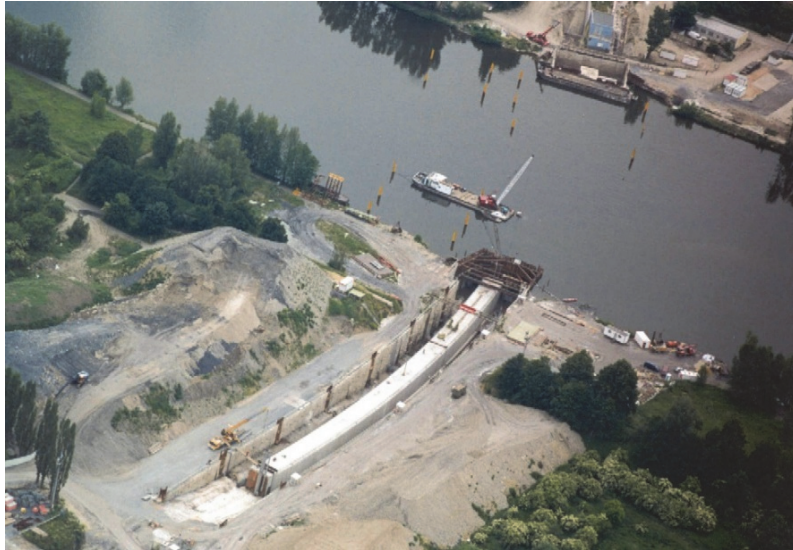
Fig. 14. Aerial view on the dry dock with the tunnel tube prepared for launching
