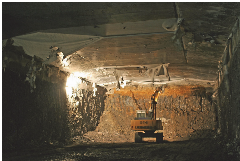
Fig. 13. Excavation works under the protection of the top slab of the tunnel
