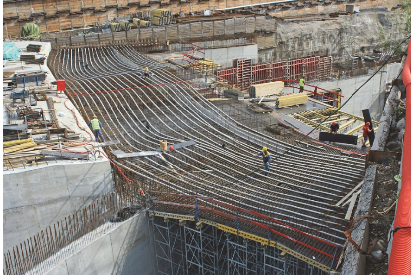
Fig. 12. Prestressing tendons assembled in the top slab of the cut and cover tunnel
